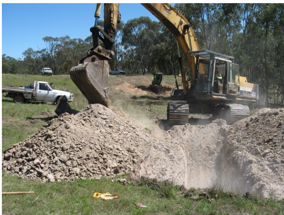
Figure 1: Excavating a bulk sample pit into the Karaula Lead alluvial tin deposit at Elsmore using a 30t excavator
