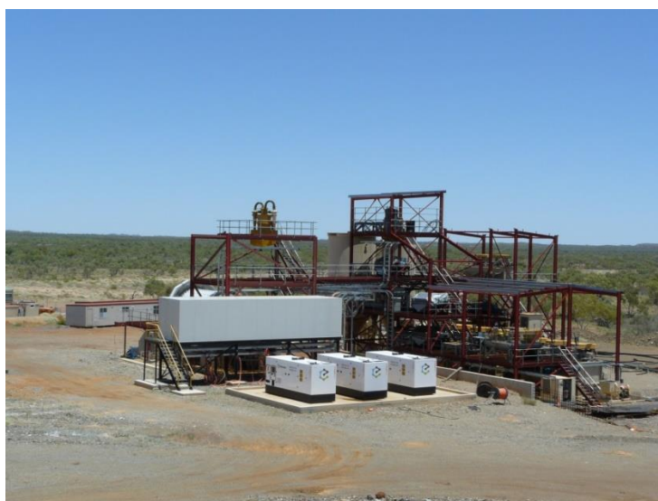
Lorena Concentrator Plant
